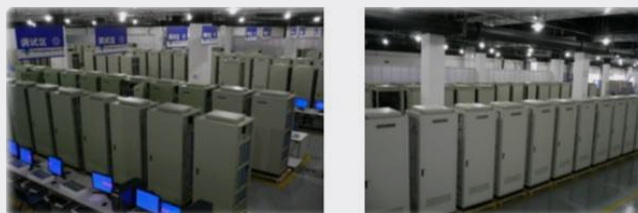
Field Control Cabinets
