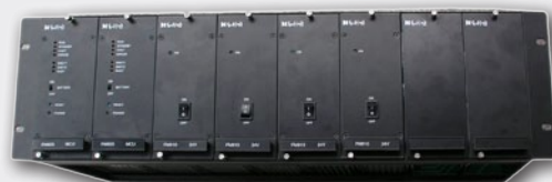
The FM Controller installed on a system rack
