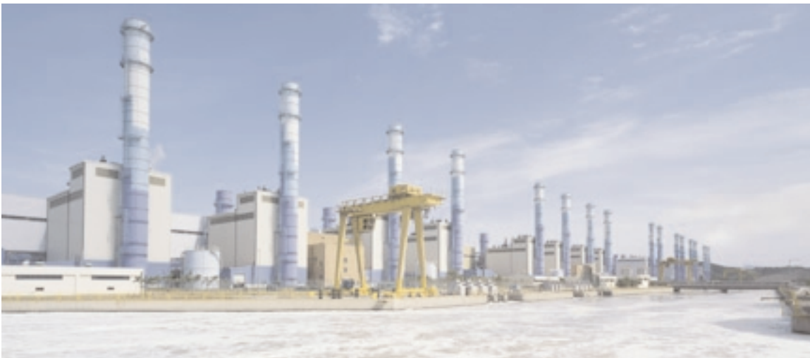
Figure 47. 4000 MW multi-shaft STAG installation
